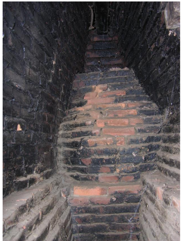
SMOKE BLACKENED CHAMBER
