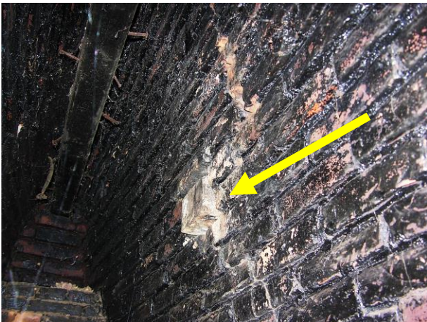
LOOSE SQUARE BRICK
